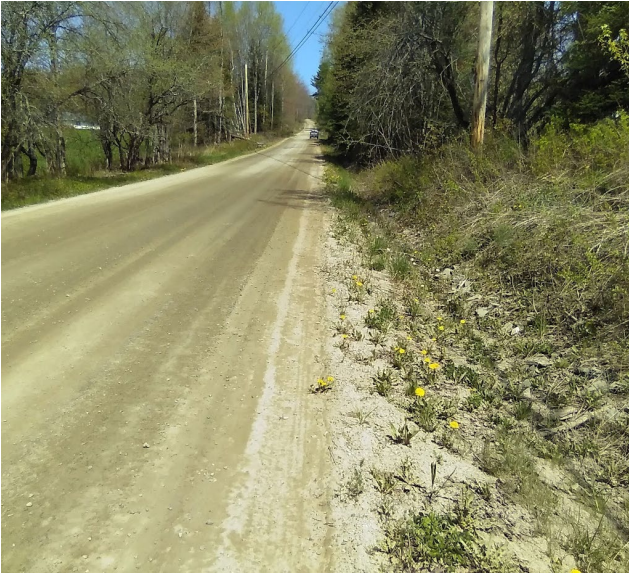
The ditches in segment 1931.1, 1932.1, and 1933.1 have filled with sediment and lack stone, causing sediment transport to waterbodies.
