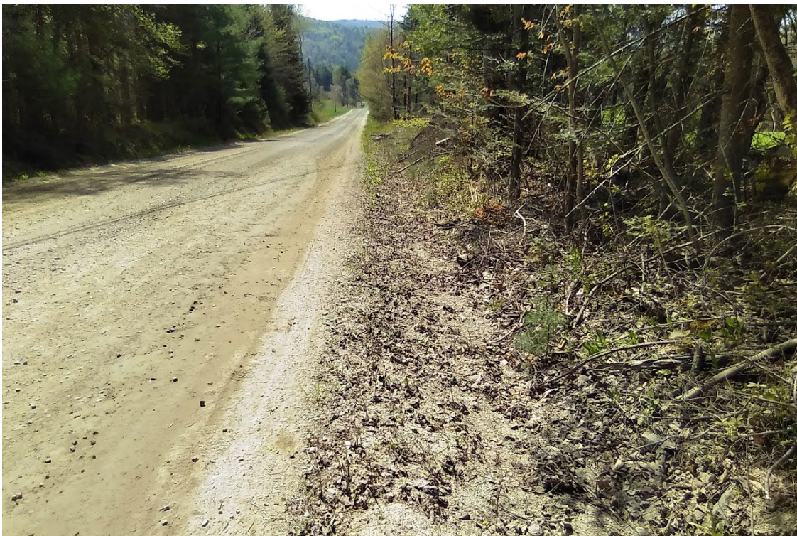
Figure 4: The ditches in segment 1931.1, 1932.1, and 1933.1 have filled with sediment and lack stone, causing sediment transport to waterbodies.
