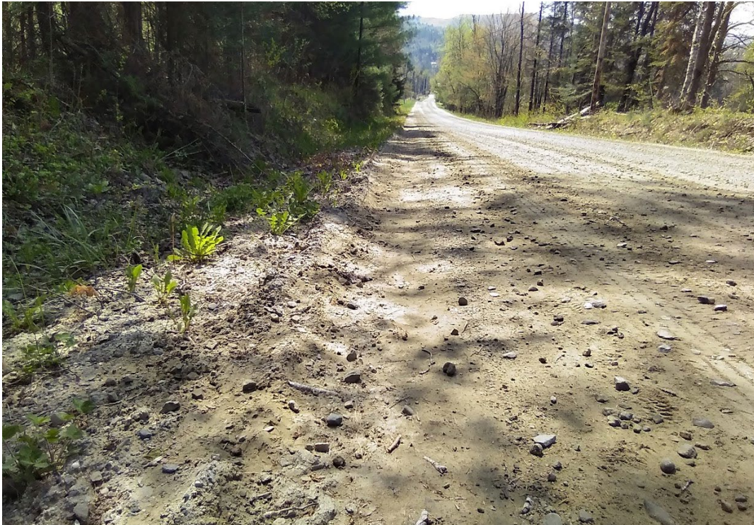
Figure 3: The ditches in segment 1931.1, 1932.1, and 1933.1 have filled with sediment and lack stone, causing sediment transport to waterbodies. Grader berms and poorly formed shoulders cause erosion on the road.
