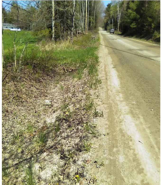
The ditches in segment 1931.1, 1932.1, and 1933.1 have filled with sediment and lack stone, causing sediment transport to waterbodies.
